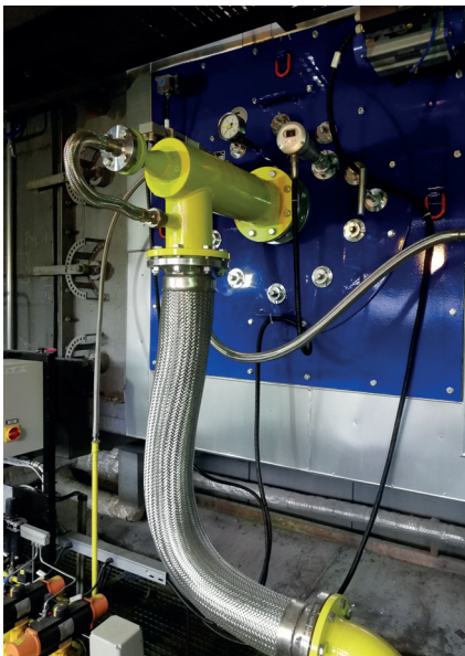
Detail of the burner
