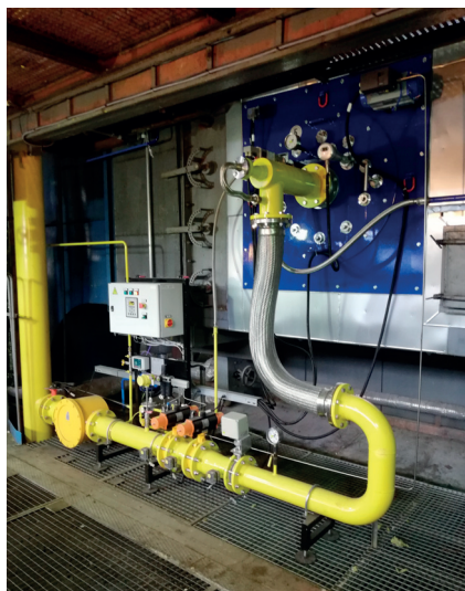
Detail of the burner with the supply of natural gas to the burner
