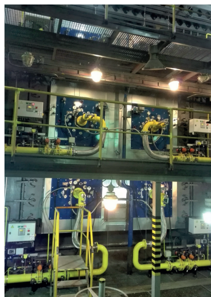
Placement of burners on three floors of a boiler with an output of 110 MW
