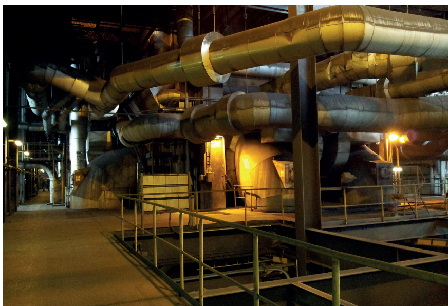
Drying tubes of a coal-fired boiler
